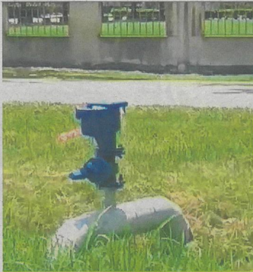
Water can be seen flowing out from the loosened valve on this main water pipe in Taman Klang Jaya.
